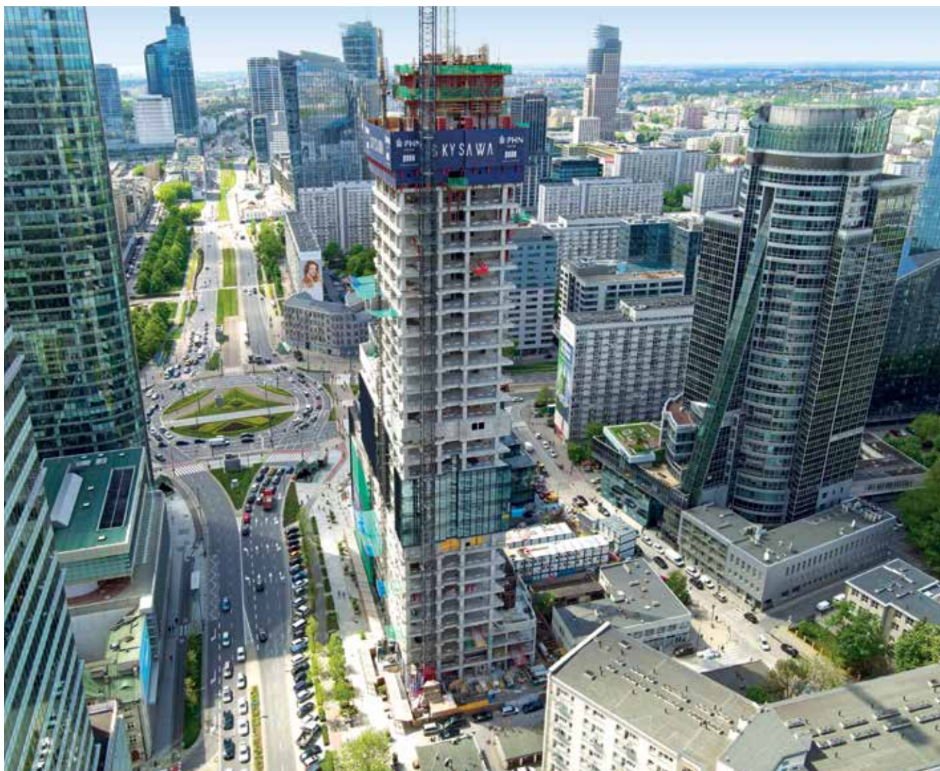
Multiple records for one tower: The 155-metre SKYSAWA pencil tower dominates the Warsaw skyline with 40 floors and a total area of 40,000m 2 . Built by PORR, which is once again setting records with future-proof technologies and a pioneering spirit.
