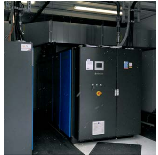
Two cogeneration modules provide the POLYTEC location in Altenstadt with a reliable, clean and favourably priced energy supply.
