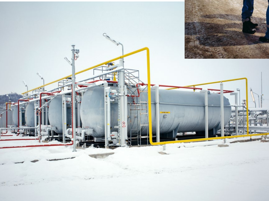
At the end of the day, all information is handed over to the night shift (top). Condensate storage vessels are positioned in a dyke for ultimate safety (left).
