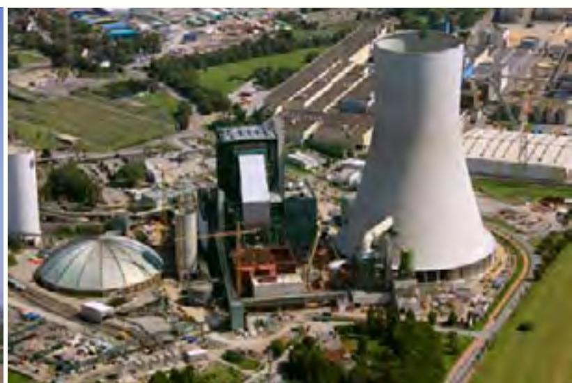
Construction of one of Europe's most modern coal-powered plants in Duisburg-Walsum, Germany
