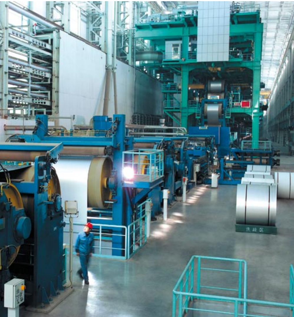
▲ Cold-rolled strip annealing and pickling line by ANDRITZ METALS for Taiyuan Iron and Steel (Group) Company Ltd., China.
