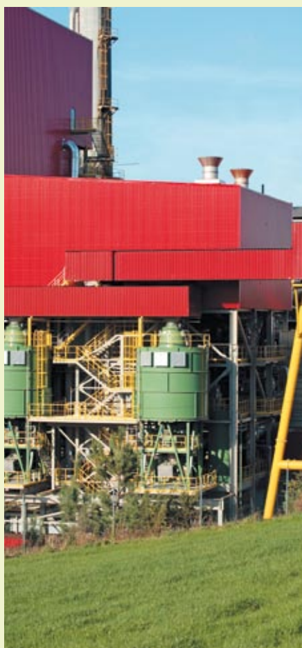
Energy from biomass: ANDRITZ biomass-fired power boiler at the ENCE mill in Navia, Spain. ▼
