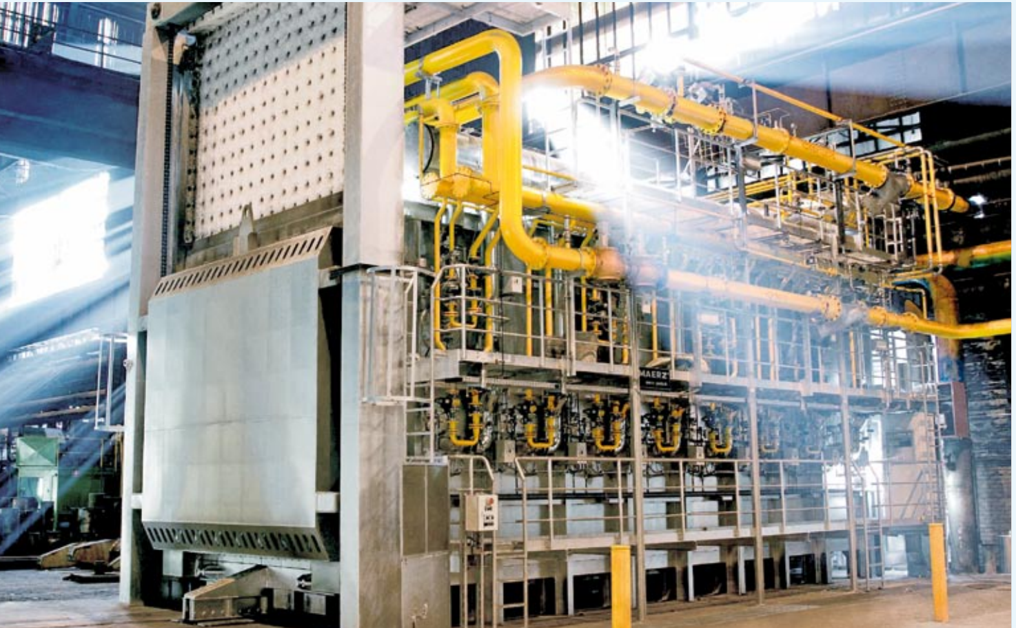
▲ ANDRITZ Maerz car bottom forging furnace for Saarschmiede GmbH, Völklingen, Germany.
